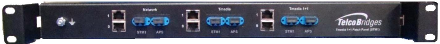
Tmedia TMG3200-STM1 1+1, Patch Panel (front view)
